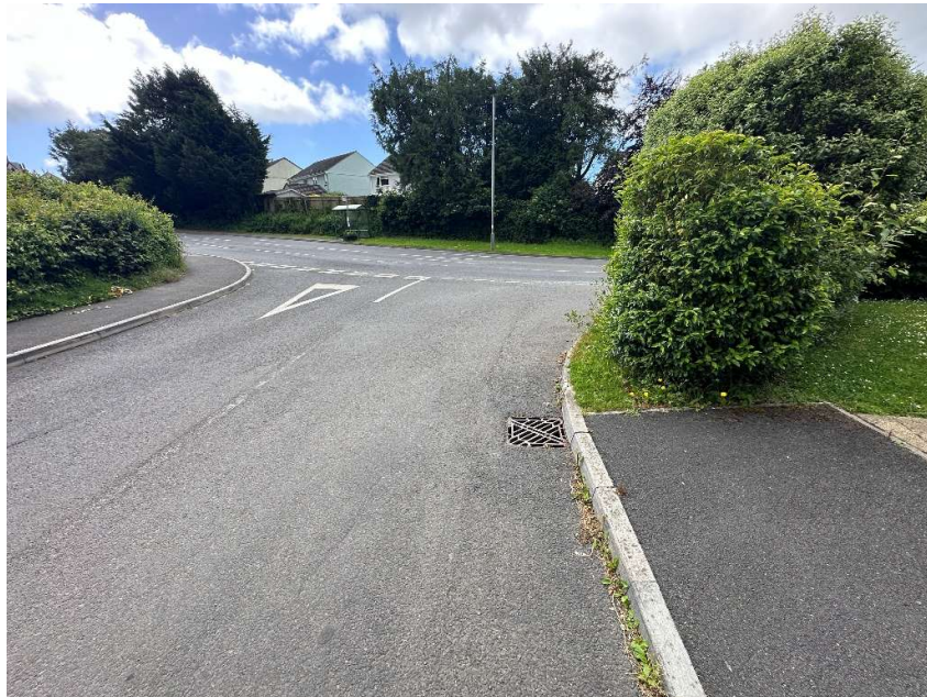
Footway Terminating Abruptly at Lanveoc Way/A379 - Aprica Image
